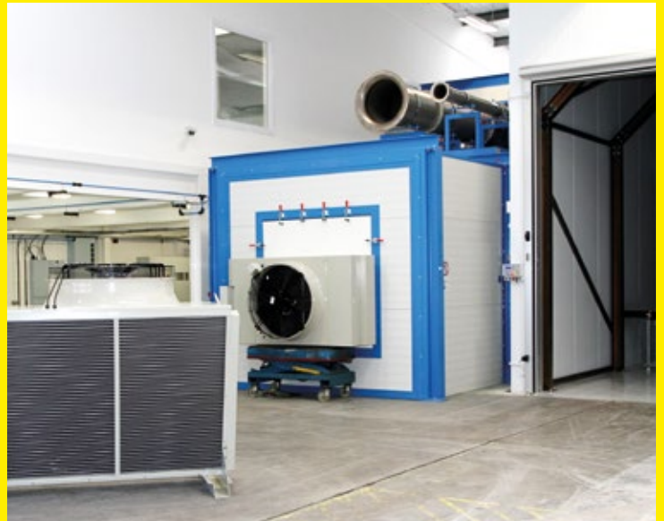
Wind Tunnel – Discharge Chamber 3m 2
